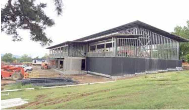
Fuhrmann Hall is progressing -- roof, exterior walls, plumbing, electrical, duct work, and mechanical.
